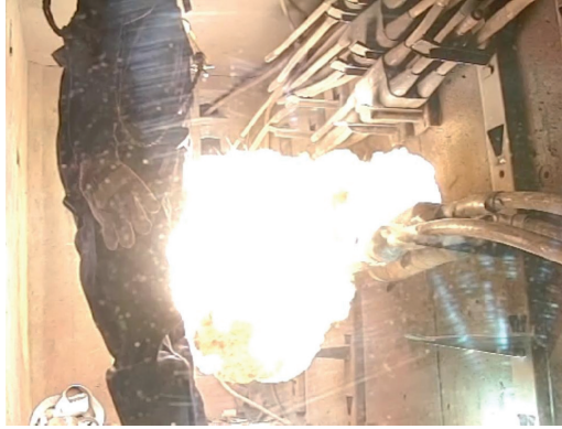
Figure 14.40 Con Edison PILC splice failure test. (From EPRI 1018693, Distribution Arc Flash: Analysis Methods and Arc Characteristics , Electric Power Research Institute, Palo Alto, CA, 2009. Copyright 2009. Reprinted with permission.)
