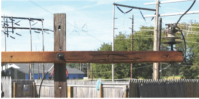
Figure 13.34 Near-surface damage from impulses. (From EPRI 1021995, Distribution Composite Crossarm Laboratory Testing , Electric Power Research Institute, Palo Alto, CA, 2011. Copyright © 2011. Reprinted with permission.)
