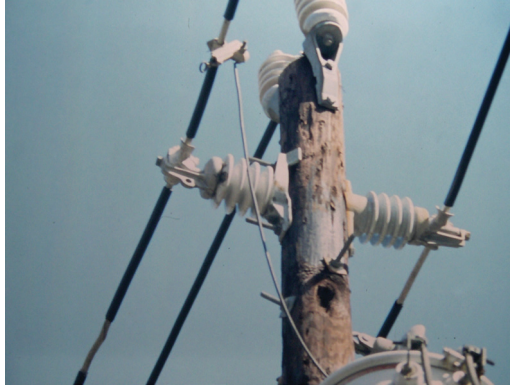
Figure 3.13 Example of a compact armless design using covered conductors. (Courtesy of Duke Energy.)
