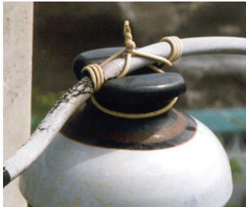
Figure 3.15 Example of a covered wire tie on a covered conductor. (From Vincent, W. R. et al., The Mitigation of Radio Noise and Interference from External Sources , 6th ed, United States Navy Naval Postgraduate School, 2007.)
