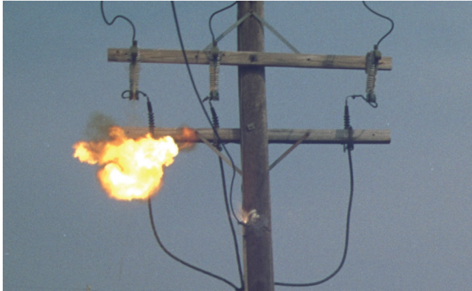
Figure 9.3 Example operation of an expulsion fuse during a fault. (Courtesy of the Long Island Power Authority.)
