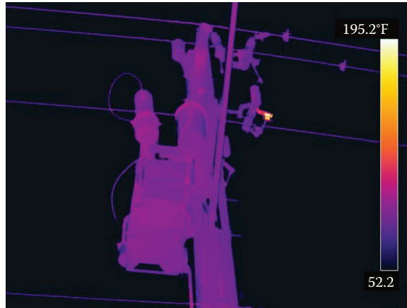
Figure 7.24 Hot capacitor cutout. Note the blown fuse on another phase. (Courtesy of Osmose Utilities Services, Inc.)
