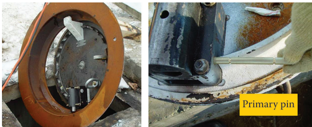
Figure 14.35 Bottom view of a manhole cover with controlled pressure relief. (From EPRI 1015889, Manhole Event Risk Management Strategies: High-Level Overview , Electric Power Research Institute, Palo Alto, CA, 2008. Copyright 2008. Reprinted with permission.)
