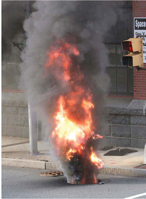
Figure 14.33 Example manhole event. (From EPRI 1015889, Manhole Event Risk Management Strategies: High-Level Overview , Electric Power Research Institute, Palo Alto, CA, 2008. Copyright 2008. Reprinted with permission.)
