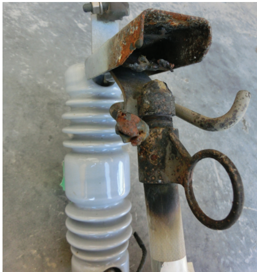
Figure 7.25 Cutout damaged by arcing in the field.
