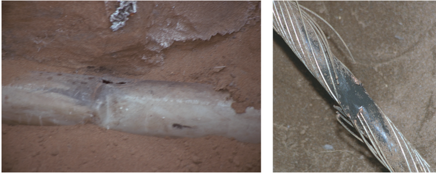
Figure 13.25 Cable and conduit damage observed from rocket-triggered lightning flashes above the ground. (From Electric Power Research Institute. Copyright © 1993. Reprinted with permission.)
