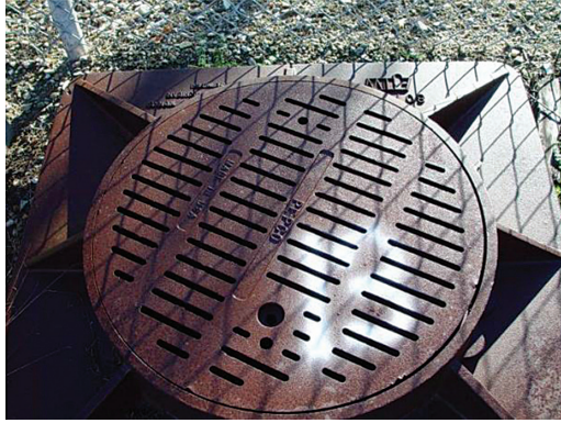
Figure 14.34 Vented manhole cover. (From EPRI 1015889, Manhole Event Risk Management Strategies: High-Level Overview , Electric Power Research Institute, Palo Alto, CA, 2008. Copyright 2008. Reprinted with permission.)
