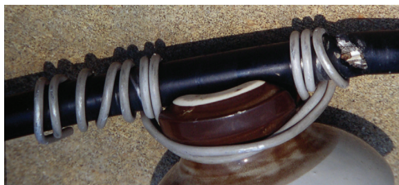
Figure 3.16 Example of damage on a covered conductor from flashover at the insulator tie. (Courtesy of Duke Energy.)
