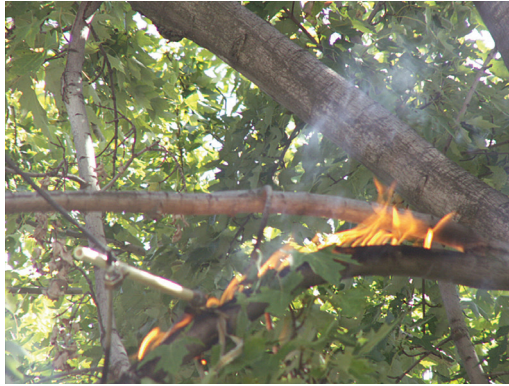
Figure 14.28 Open flame on a silver maple branch energized at 7.6 kV. (From EPRI 1016219, Optimal Design of Overhead Distribution Systems: Understanding Touch Voltage Potential Risks Due to Tree-to-Conductor Contacts on Distribution Circuits , Electric Power Research Institute, Palo Alto, CA, 2007. Copyright 2007. Reprinted with permission.)
