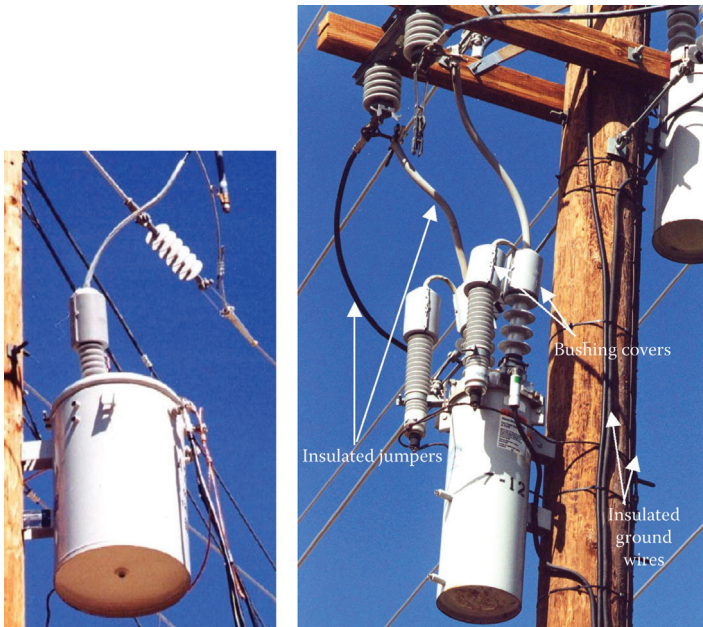
Figure 3.18 Examples of wildlife protection with animal guards and covered jumpers. (From EPRI 1001883, Distribution Wildlife and Pest Control , Electric Power Research Institute, Palo Alto, CA, 2001. Copyright 2001. Reprinted with permission.)
