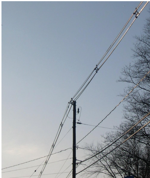
Figure 2.4 13.2-kV spacer cable.
