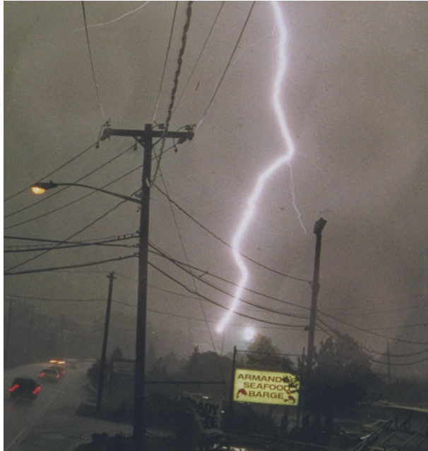
Figure 13.31 Lightning-caused fault on a Long Island Lighting Company 13-kV circuit. (Short, T. A. and Ammon, R. H., Monitoring results of the effectiveness of surge arrester spacings on distribution line protection, IEEE Transactions on Power Delivery , vol. 14, no. 3, pp. 1142–50, July 1999. © 1999 IEEE.)
