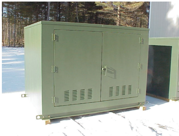
Figure 7.3 Example padmounted capacitor. (From Northeast Power Systems, Inc. With permission.)
